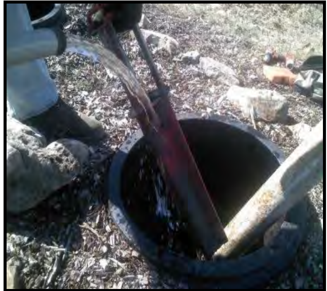
Properly cleaning a dirty EFFLUENT screen.
