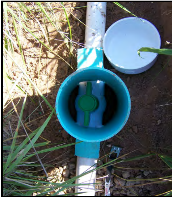
Low Pressure Pipe Valve (LPP). Valve opened to flush LPP distribution line. After flushing, valves are used to adjust the operating pressure in each LPP distribution line.
