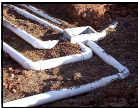
Concrete distribution box
