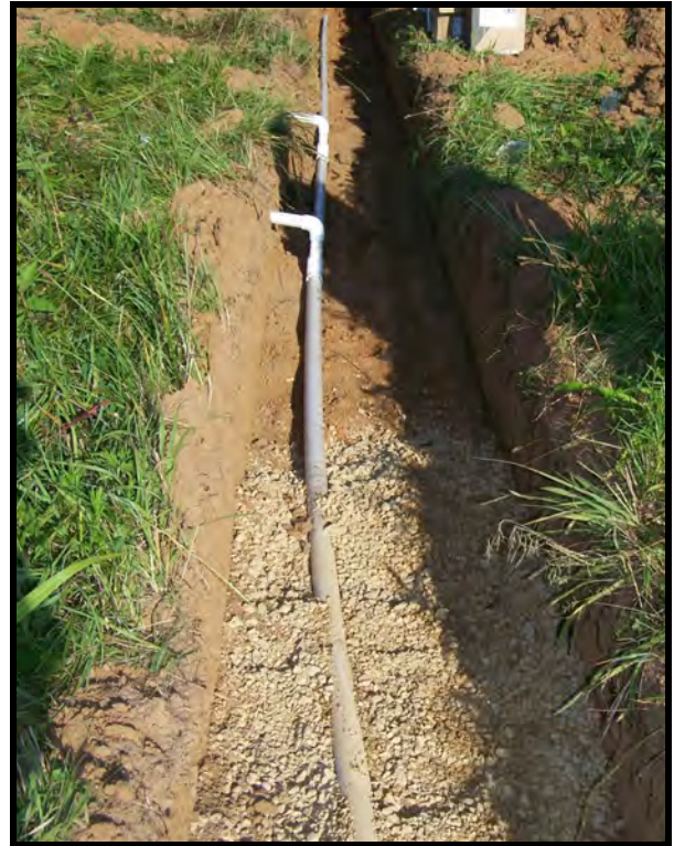
Low Pressure Pipe Manifold. The manifold trench and connections to LPP valves and distribution lines.
