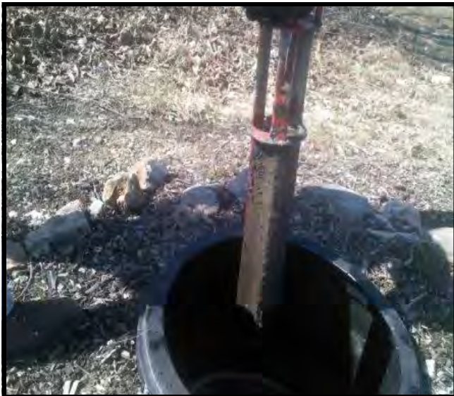
A dirty EFFLUENT screen. This screen is located in the outlet baffle of a septic tank.
