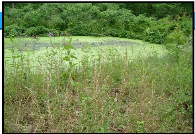
Lagoon MAINTENANCE includes cutting grass, weeds, and trees growing near the lagoon. The lagoon berm can be damaged when woody plants are allowed to grow. Duckweed growing on the water surface and grass or weeds growing over the waters edge can interfere with treatment and harbor mosquitoes.
